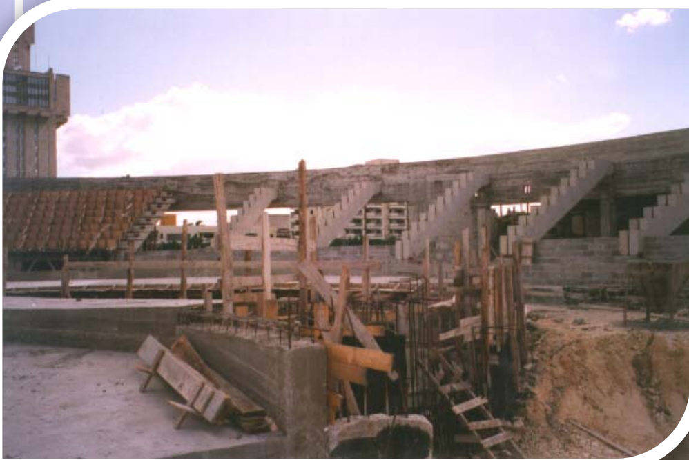
Waterproofing and protection of stands in Dolphin show area in National Aquarium (Cuba)
